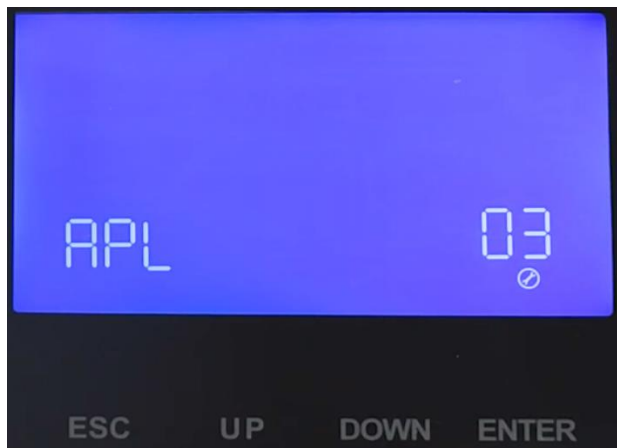
Figure 2.1.5.7 Growatt operation panel
