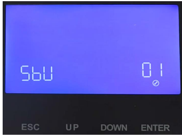
Figure 2.1.5.6 Growatt operation panel
